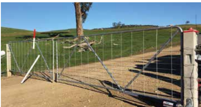
First solar gate to be installed on the project. The process has been refined to include a sliding bar on the offside gate to provide greater security. ■
