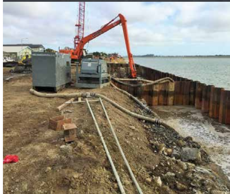
Above top: The rebuilt section of the seawall is 500m in length and runs beside the new Christchurch Coastal Pathway.
