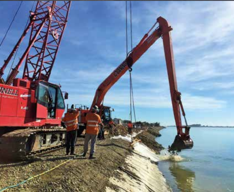
Above: Two layers of rock are placed along the exterior of the seawall to provide additional protection.
